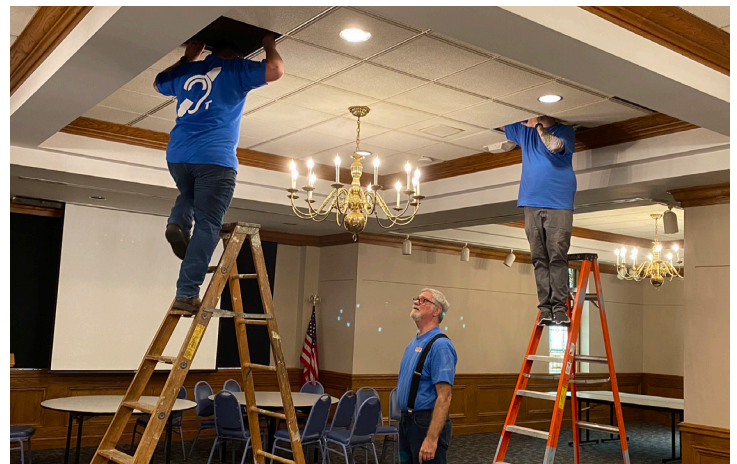
Below: Brown Audio Service, LLC installs the hearing loop for the Upper Room via the Fellowship Hall ceiling.
